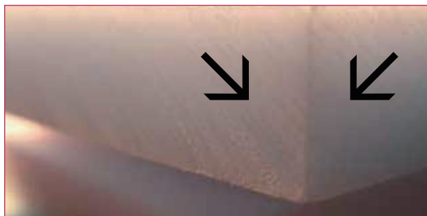
pic. Shows marks from the saw blade.
