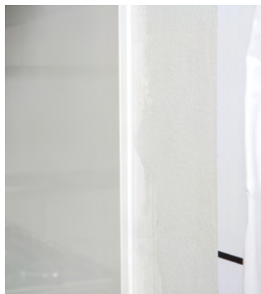
Figure 2: Metaline splashback butted against a wall showing use of sealant in the expansion gap.
